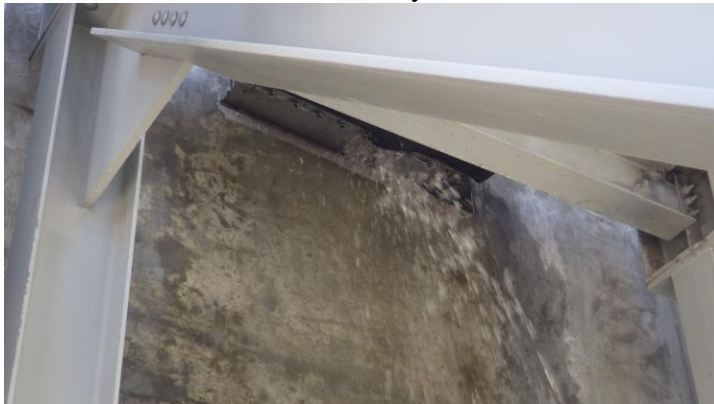
Photo 1. Expansion joint leak between the PDW and the transport flume.
